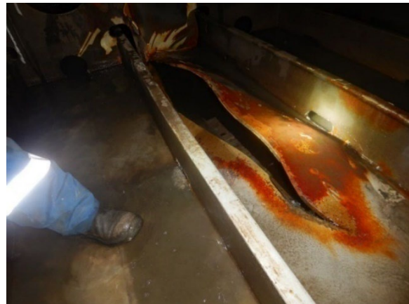
Figure 4. Damage to the vessel, viewed from inside No. 3 starboard ballast water tank (Source: Coastal Shipping Limited)
