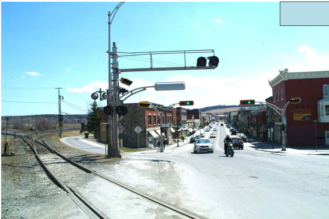
Figure 12: Curve and Switch Track Section with Depressed Rail Joint Defects
