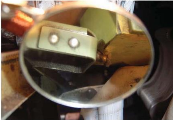
Figure 1 Stop Bolt Caught on Weight
