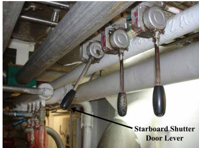
Photo 3. Hydraulic lever in the “close” position
