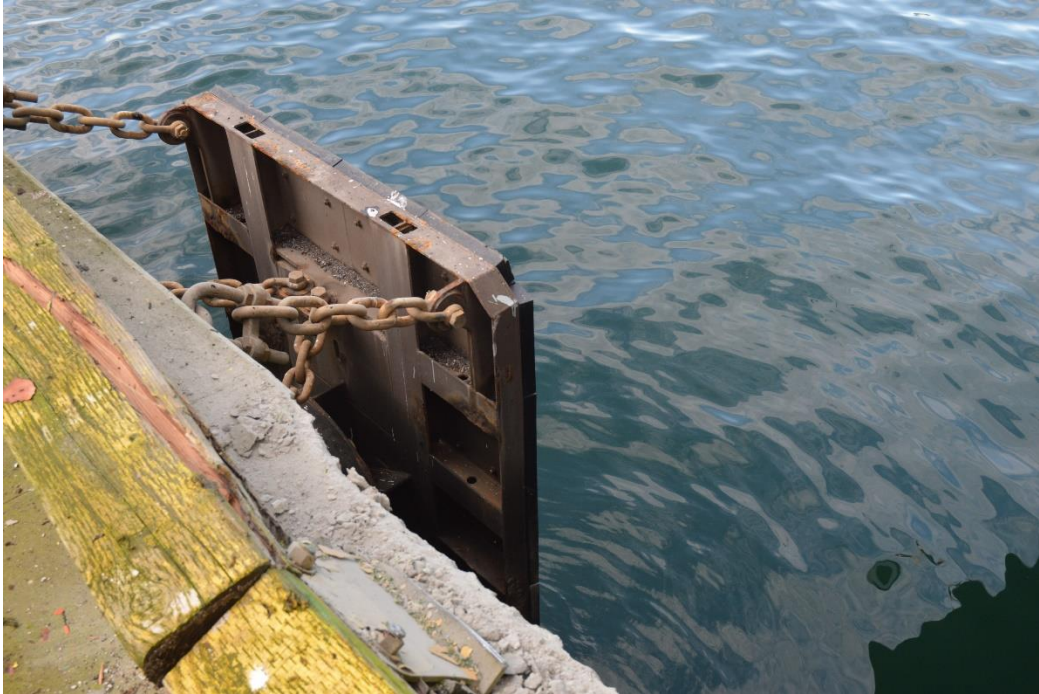
Figure 9. Cone fenders on Vanterm berth 6 extension (Source: TSB)
