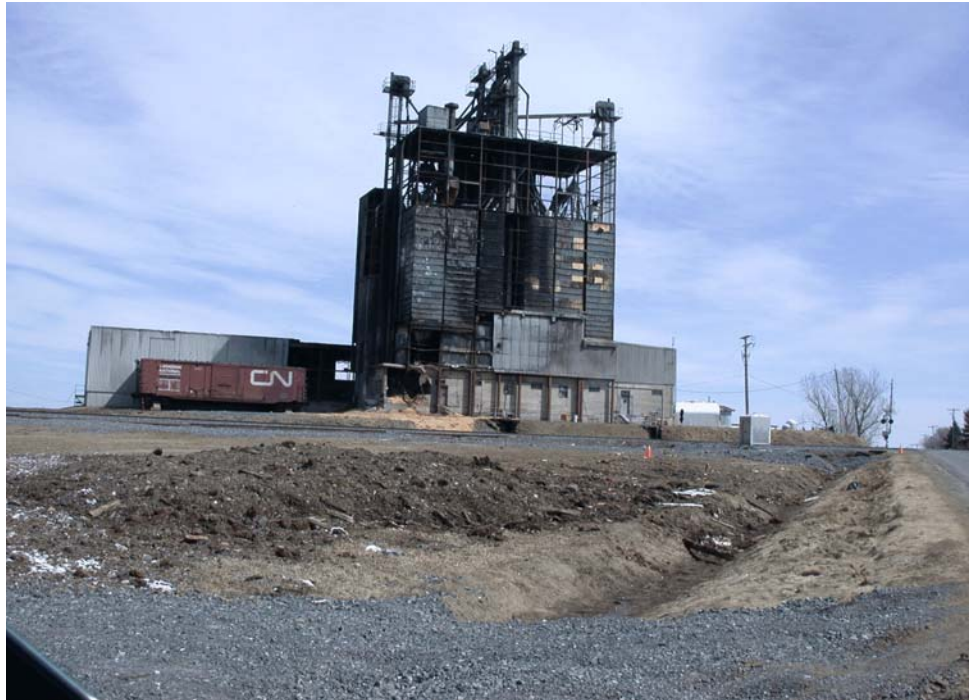
Photo 1. Damaged facade of the mill (photo taken two months after the accident)
