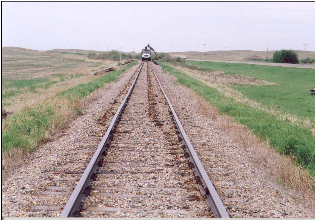
Photo 1. Point of derailment (Mile 17.4)
