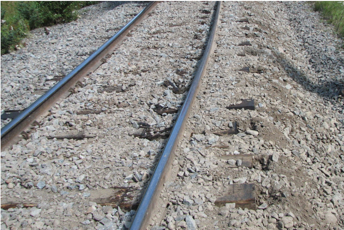
Photo 1. Disturbed ballast at ends of ties
