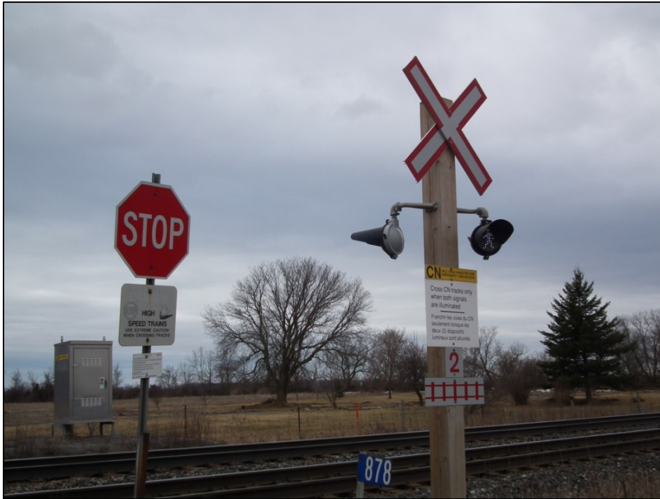
Photo 5. Walk light grade crossing warning system installed on Kingston Subdivision
