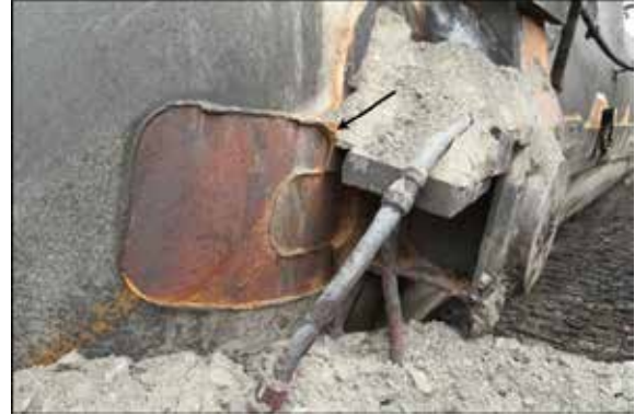
Photo 18. Damaged stub sill
