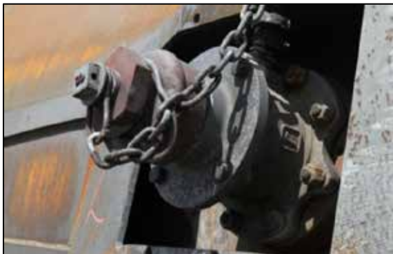
Photo 25. Bottom outlet valve
