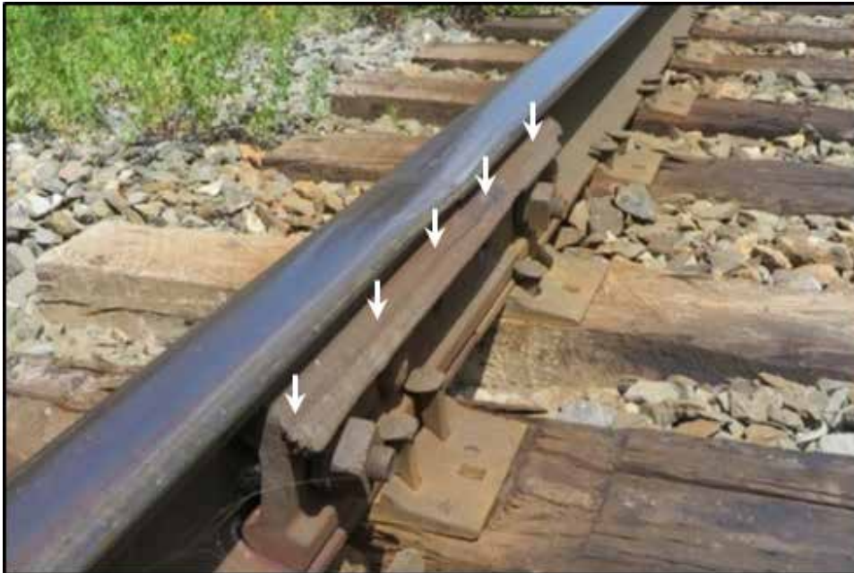
Photo 15. Damaged rail joint bar due to contact with wheel flanges
