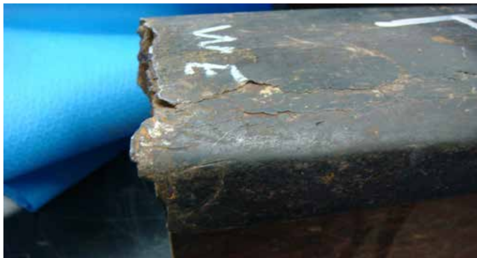
Photo 5. Rail surface conditions
