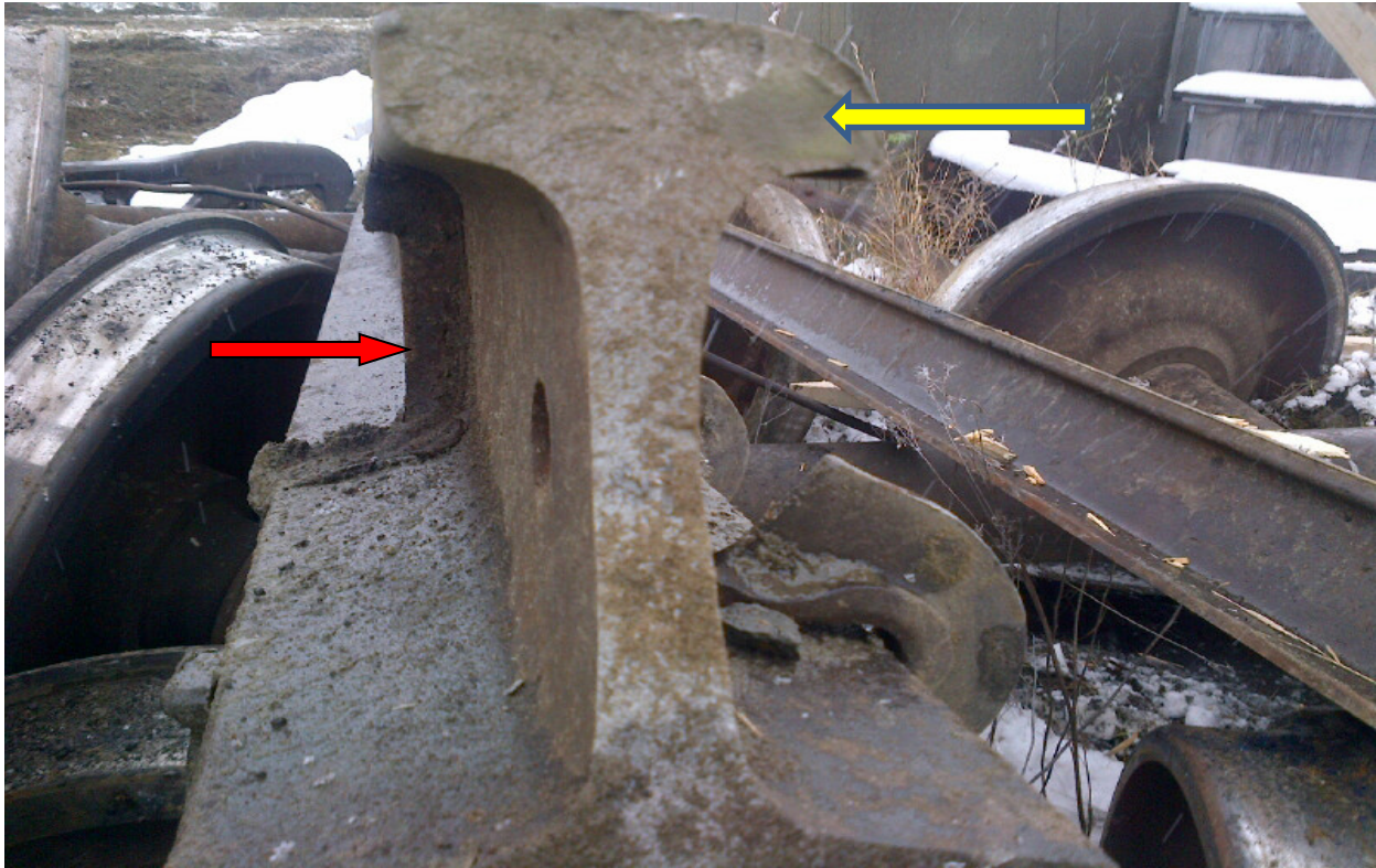
Photo 10. Transverse detail defect (TDD) in gauge corner of high rail (east end of plug [yellow arrow]) in Peers siding (note location of thermite weld [red arrow])
