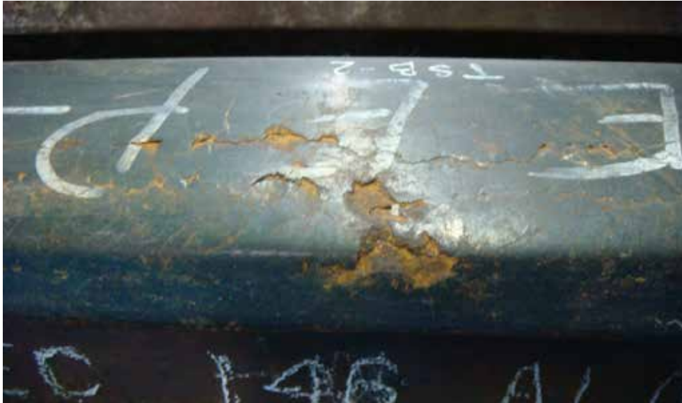
Photo 6. Rail surface conditions
