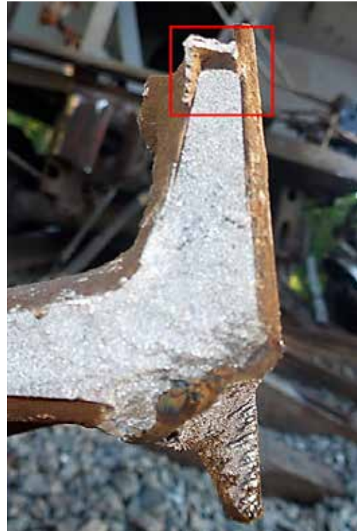
Figure 4. Close-up of the failed thermite weld's fracture surface with the origin highlighted
