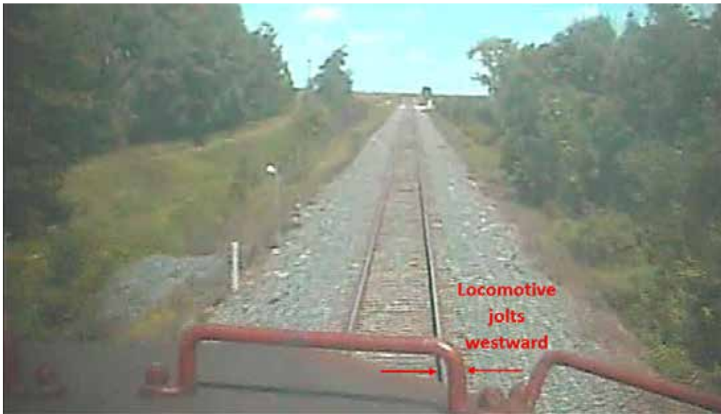
Figure 7. Locomotive jolts westward at the location of the misalignment in the west rail, with arrows highlighting the shift, as compared to Figure 6 (Source: Canadian Pacific Railway, with TSB annotations)
