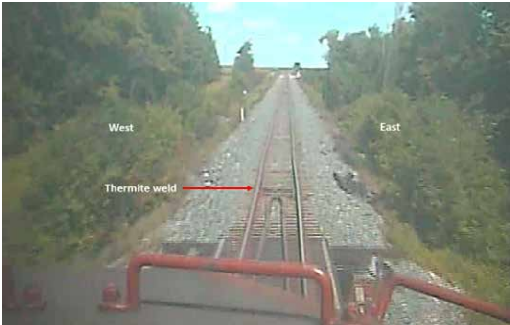
Figure 5. Thermite weld in the left (west) rail just beyond the guard rails that extended off the north end of the bridge (Source: Canadian Pacific Railway, with TSB annotations)
