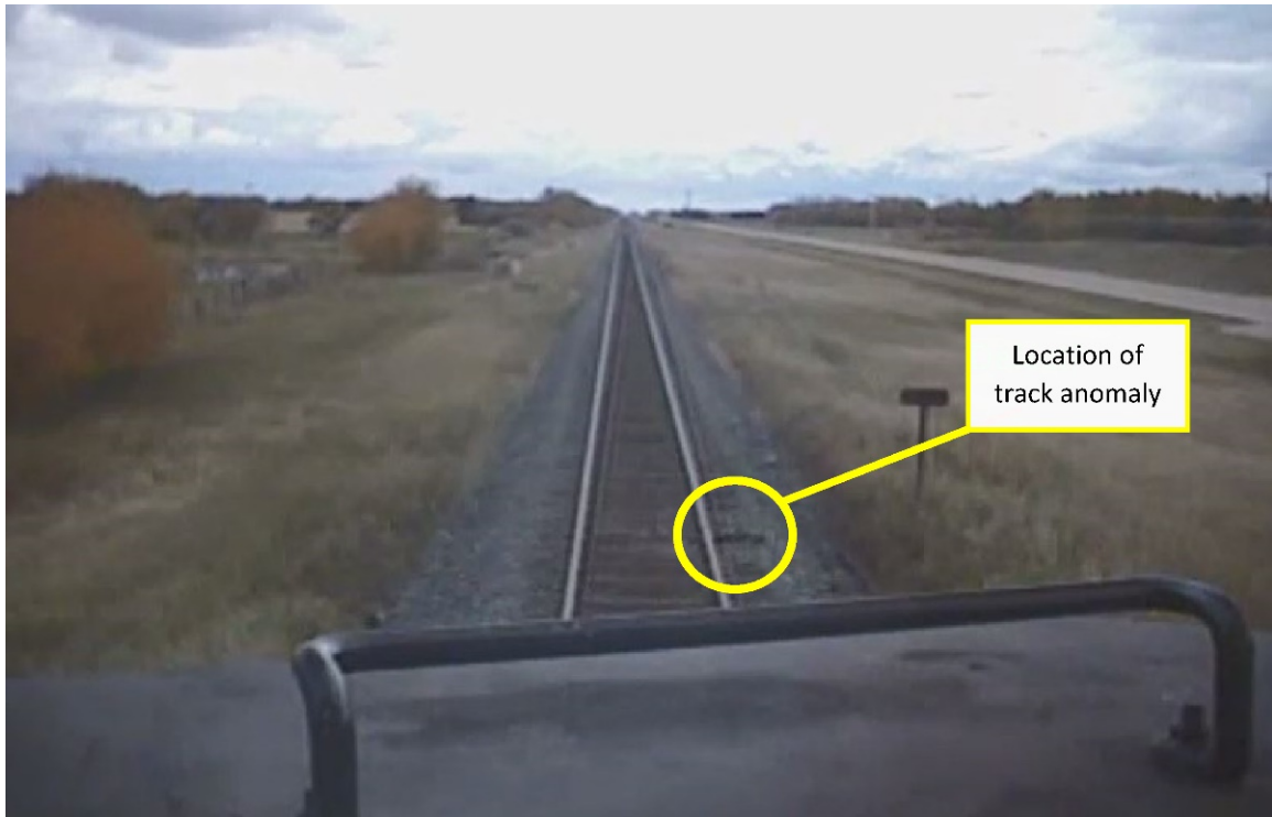
Figure 3. Forward-facing camera view of the point of derailment from a previous eastbound train, showing the track anomaly (Source: Canadian National Railway Company, with TSB annotations)
